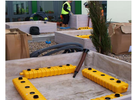
Water storage tanks and filler pipe
