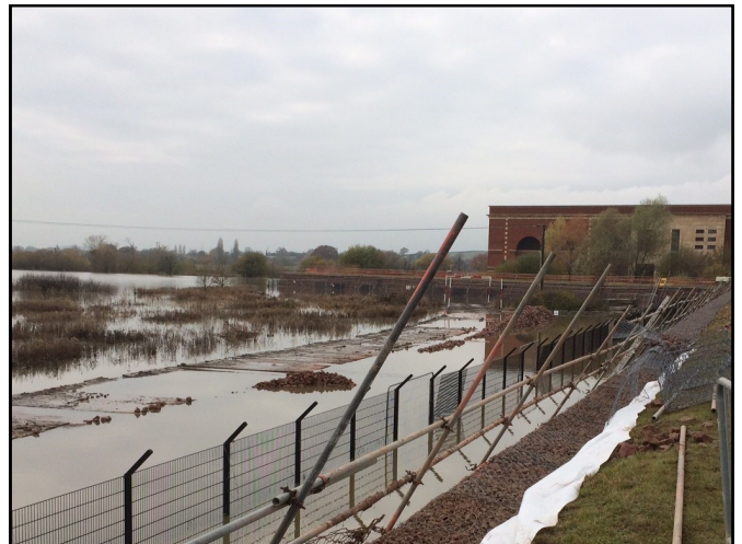
Flooding of the site during the repair works - Nov 2016
