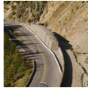
1 Rockfall and Landslide Embankments
