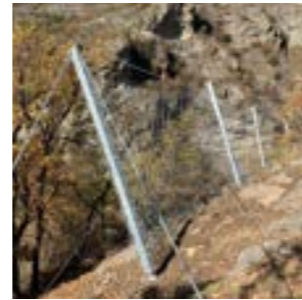
5 Dynamic Rockfall Barriers
